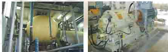
紙料工程/paper material preparation
